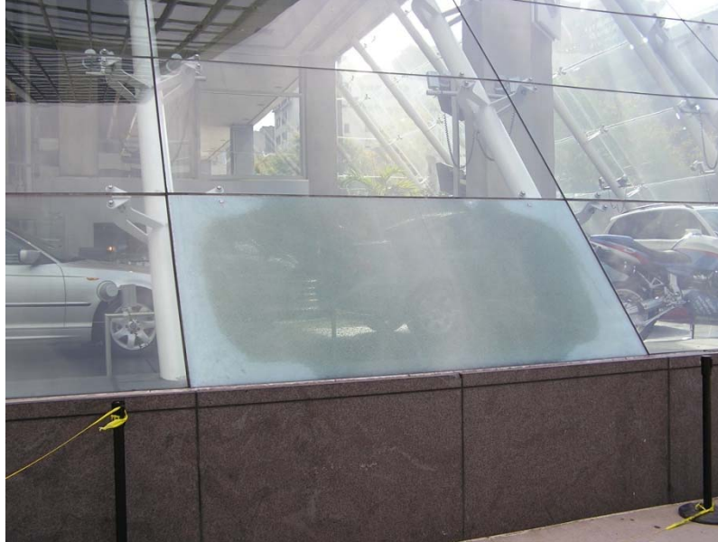
Figure 6: A laminated glass is intended to stay in frame when broken, and prevent simultaneous breakage of plies of glass. Glass laminate becomes foggy when stretched, indicating the areas stressed after breakage of both plies. New York City.
