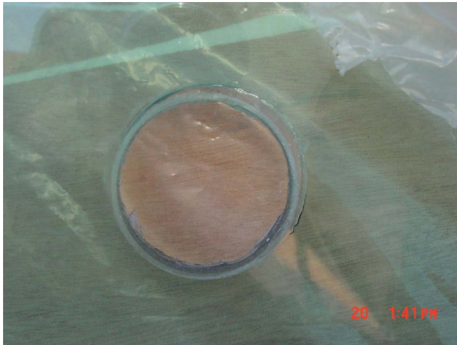
Figure 7: Laminated glass is characterized by poorer dimensional tolerances than other types of glass. However, this fact is seldom accounted for a glazing design when a standard framing is used, resulting in glass edge contamination.
