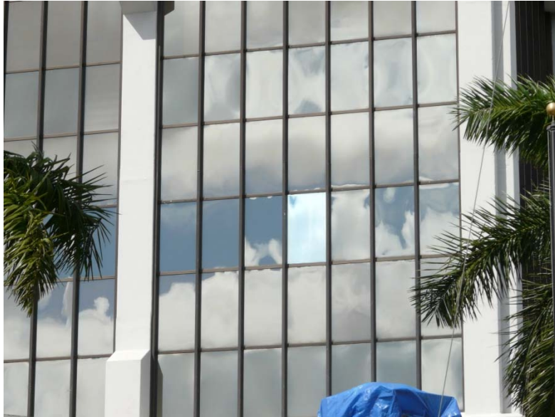
Figure 4: A typical glass mismatch caused by the lack of correct specification in a replacement glass procurement process. Miami.
