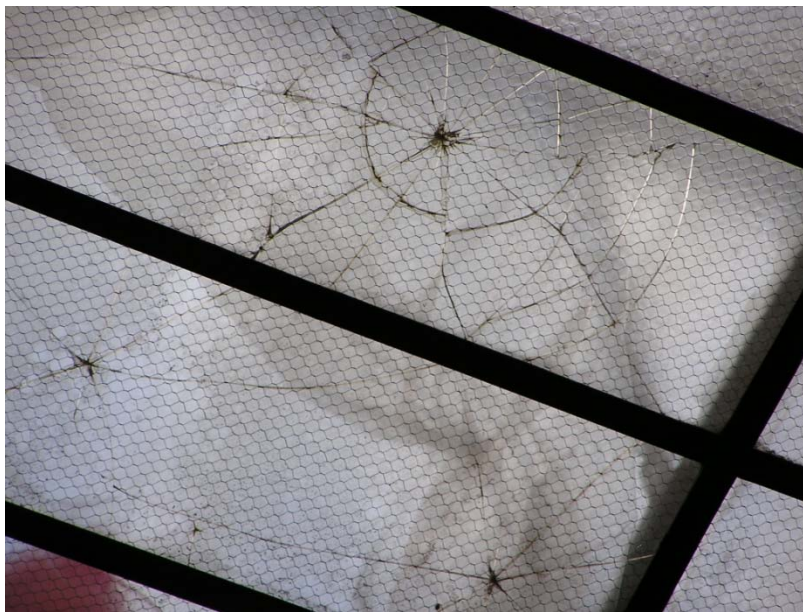
Figure 5: A laminated glass is intended to stay in frame when broken, replacing a wired glass previously used in such applications.
