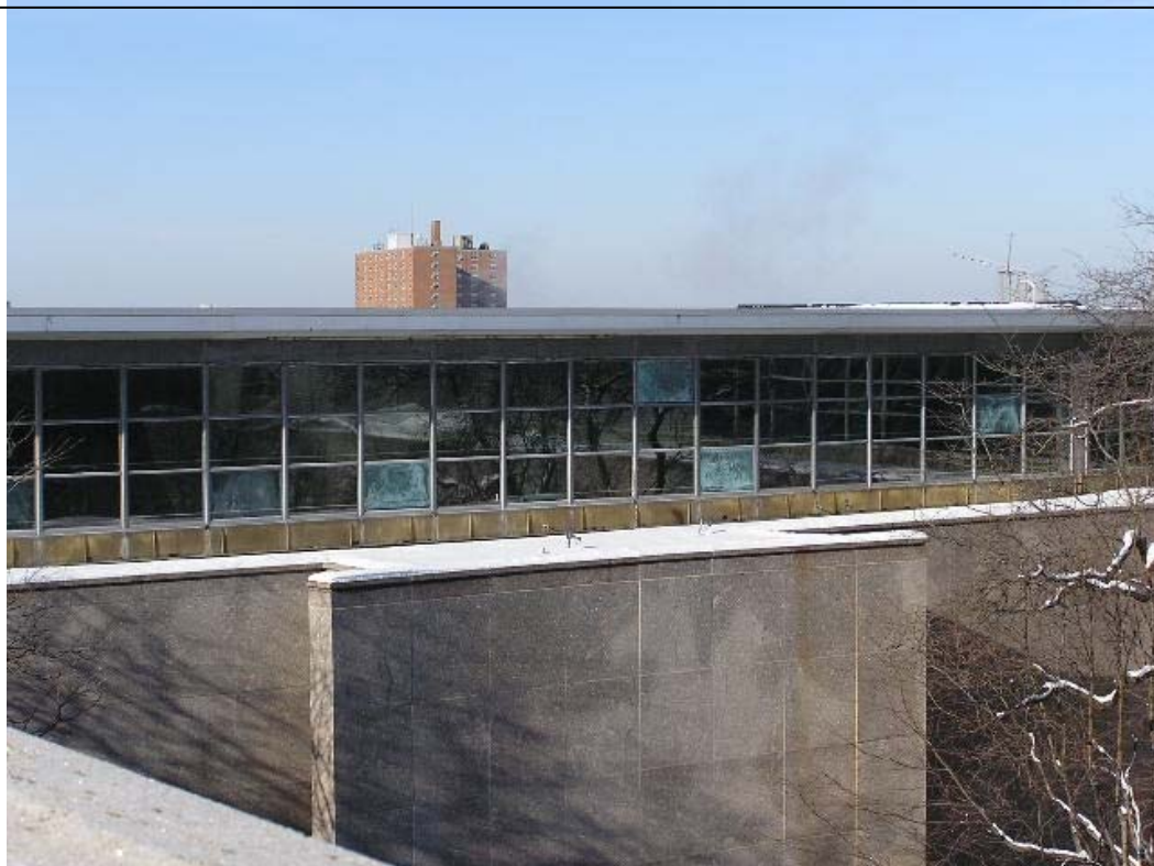
Figure 3: Frosting observed in failed insulated glass units on a facade. The Cleveland Museum of Art in Cleveland, OH.
